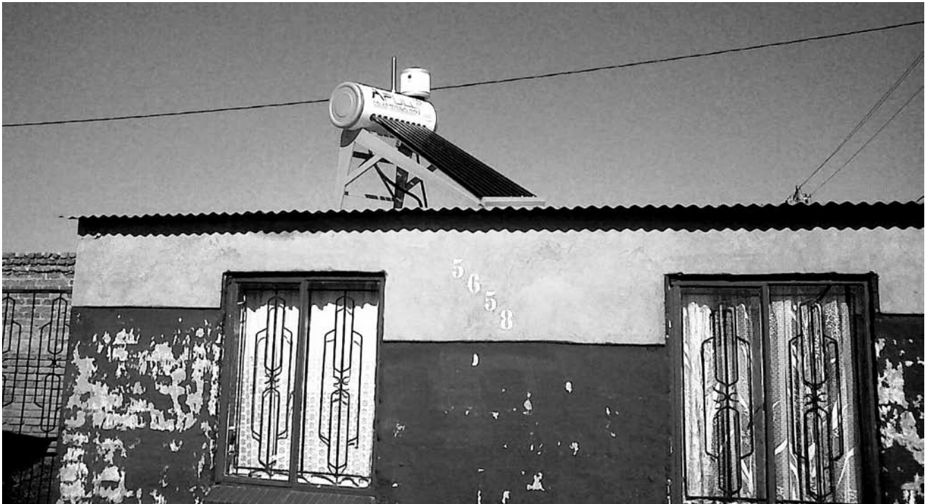
Hot water: One of the 400 000-plus solar water heaters installed free for poor households since 1994
